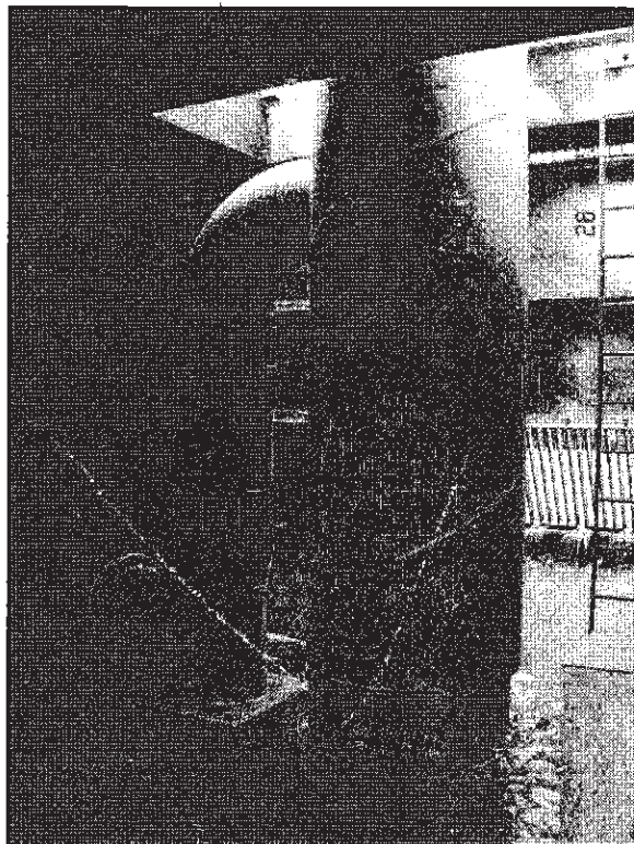
One of the new pump canisters and discharge pipes installed in the sump of Clay Lake Pumping Station.
